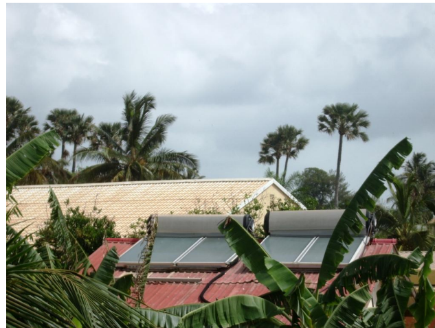
Solar water heating in locally-owned hotel
